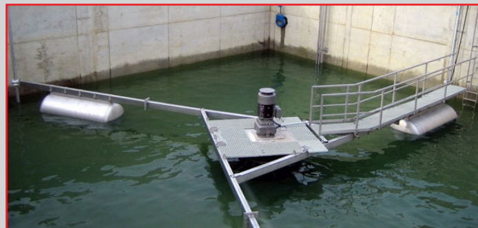
Sewage treatment plant
